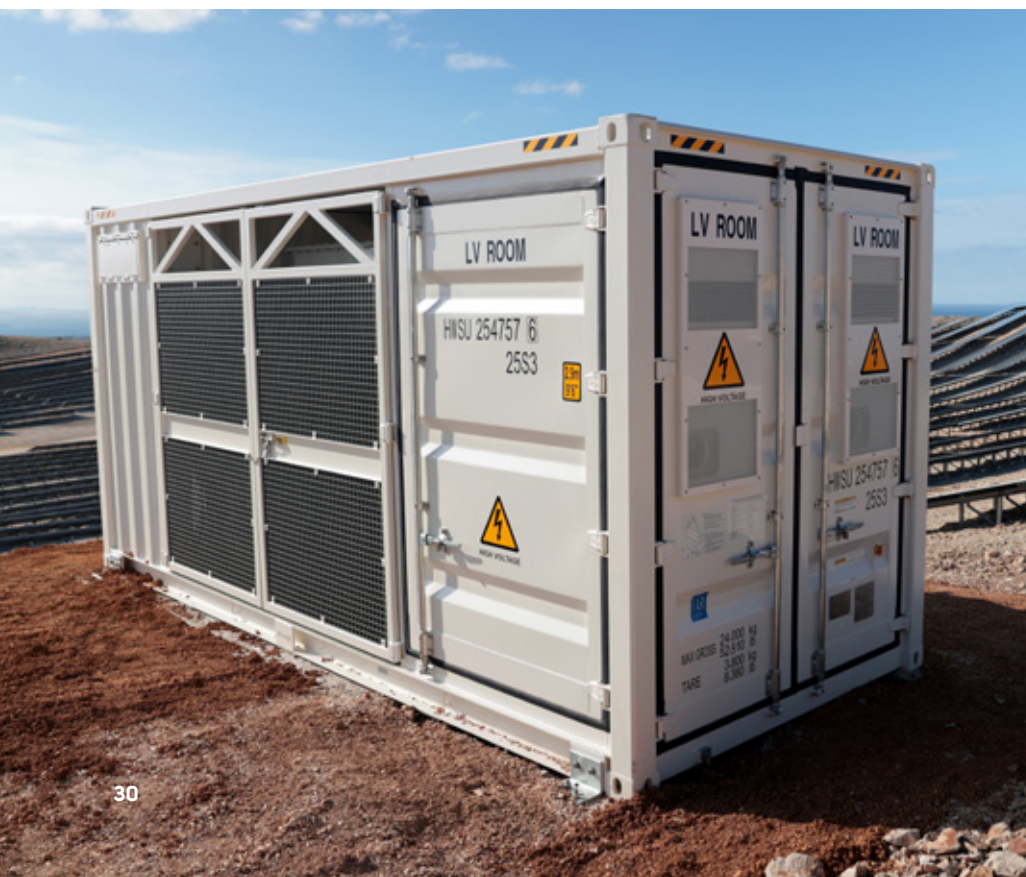
Montirane trafostanice osiguravaju stabilan prenos energije u mrežu | Installed substations ensure stable power transmission to the grid
